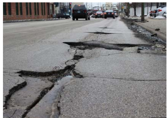
This past winter was particularly rough on road surfaces and they in turn were rough on auto alignments!
